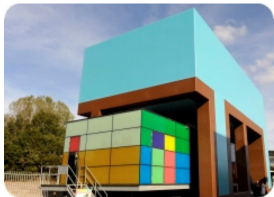
Onderstation Amsterdam RAI
