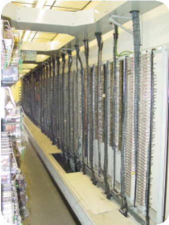
Central relay room
